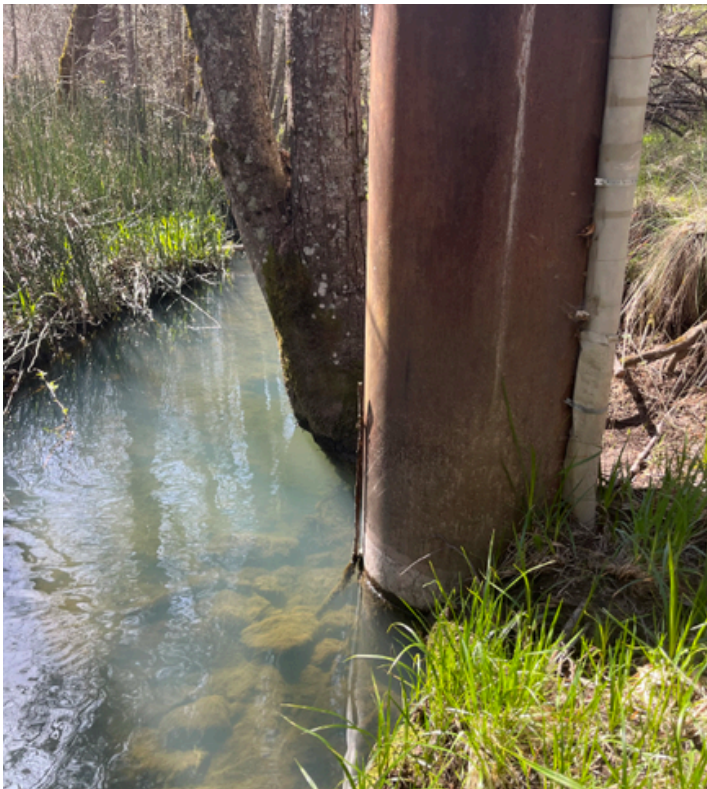
Photo of Creek Intake System
