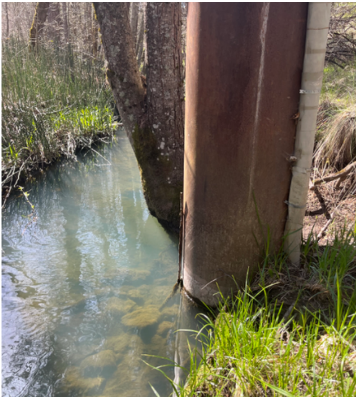
Photo of Creek Intake System
